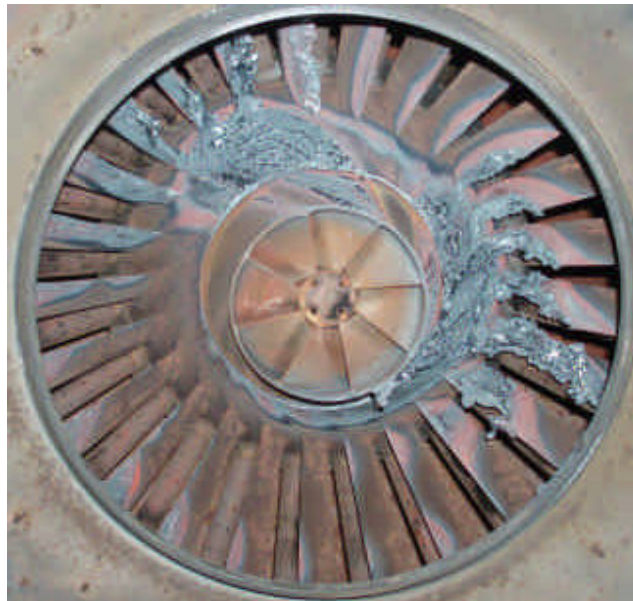
Figure C.3 – Burner Damage Caused by Flashback
